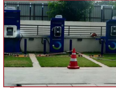
EV charging infra for employees
