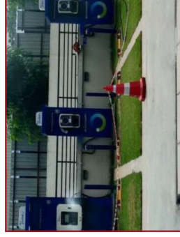
EV charging infra for employees
