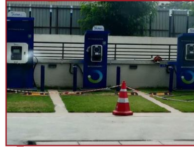
EV charging infra for employees
