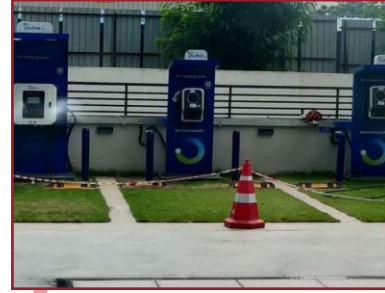
EV charging infra for employees
